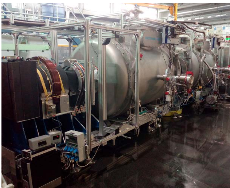
The new superconducting main precession coils in their cryostats in place at the J-NSE.
