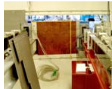
Figure 1.7: Closing the 80cm thick casemate wall towards the NG hall. Between the lead jacketed NG and the high density concrete blocks (brown) are visible the light-grey steel containers, filled with concrete, which are precisely fitted into the remaining gaps. On the left side the steel plates for final closure can be seen.
