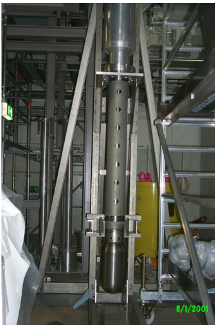
Figure 1.17: In-Pool assembly of the hot neutron source
