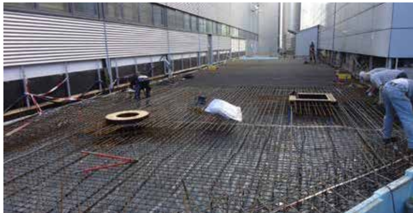
Figure 3: Construction works for the connection between the reactor building and the neutron guide hall east.
