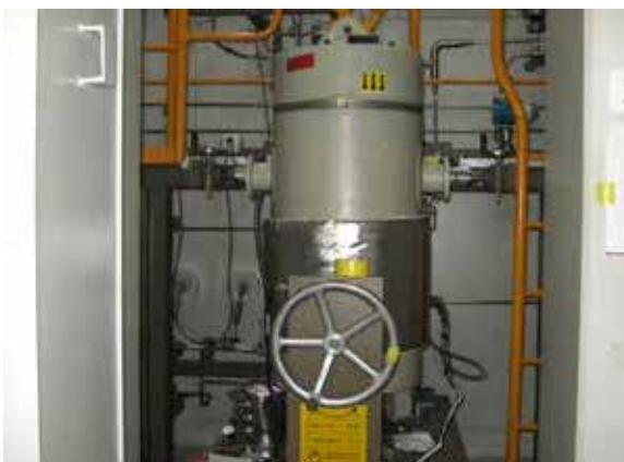
Figure 1: Ion exchange filter of the heavy water system with a heating jacket for the drying of the ion exchange resins.
