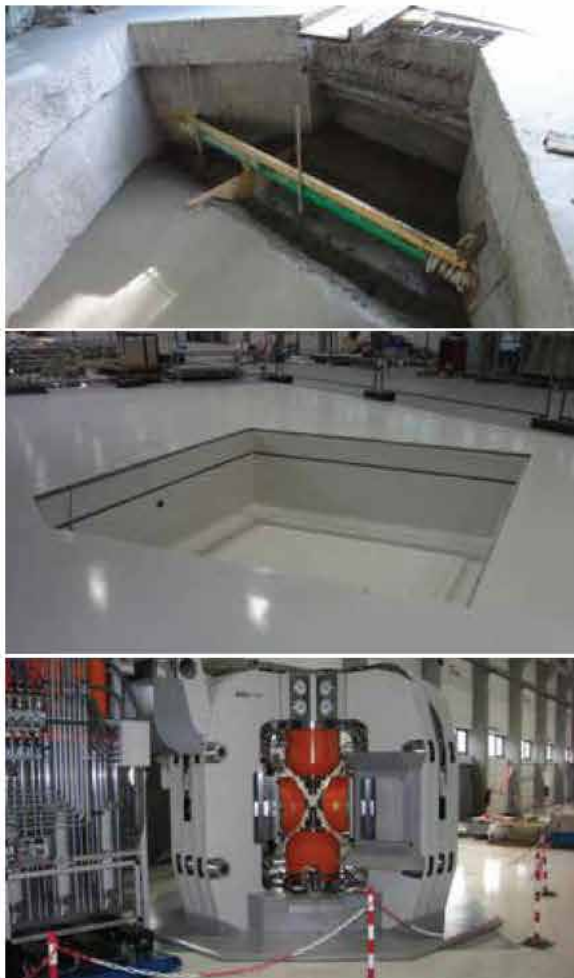
Figure 8: Floor deepening in the neutron guide hall east for the instrument SAPHiR; top: during structural work, middle: finished, bottom: with instrument installed.
