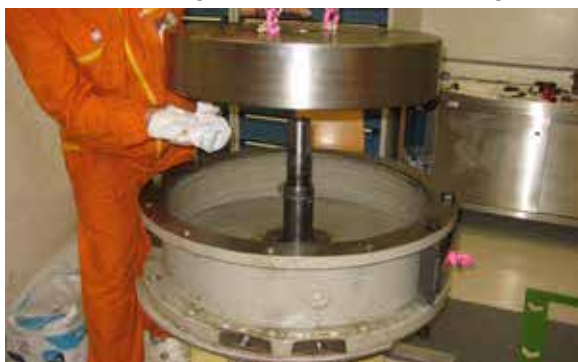
Figure 2: Removal of the flywheel for the exchange of a bearing at a primary pump.
