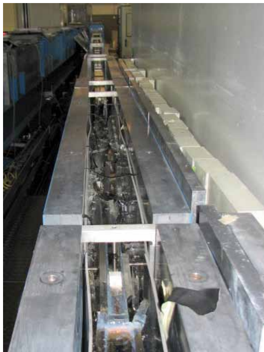
Fig. 1: View along NL5, the broken element in the foreground.
